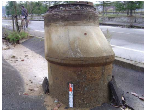
Fig. 5.1 Uplifted manhole after the 2004 Niigata-ken Chuetsu, Japan, earthquake.
