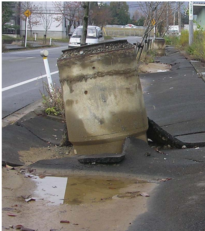
Fig. 1.1 Uplifted manholes and settlements of sidewalk after the 2004 Niigata-ken Chuetsu, Japan, earthquake.
