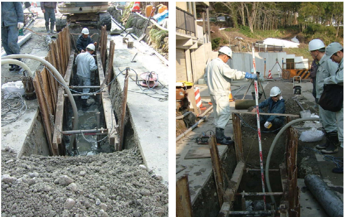
Fig. 5.3 Open-cut and level survey carried out before the restoration in Nagaoka (Nagaoka city government).
