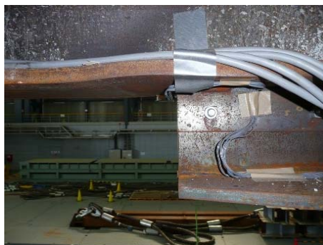
Figure 6.19 Fracture situation of connections (SL)
