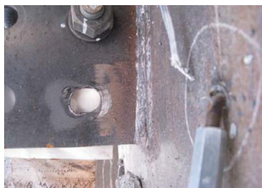
Figure 4.8 Deformation of bolt hole
