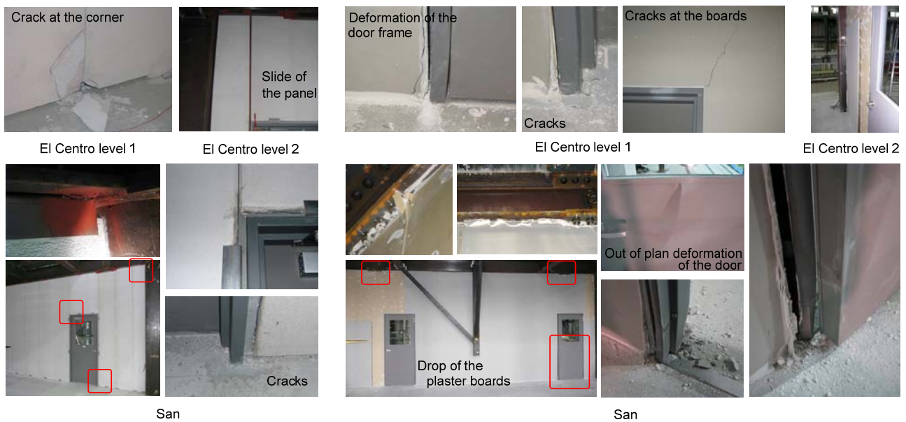
Figure 3.15 Damage to various nonstructural components
