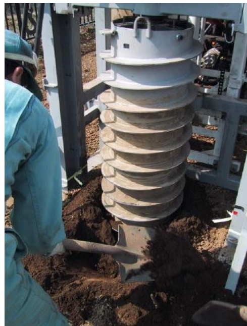
f) Press the drill down with rotation; Removal of the soil on the plane
