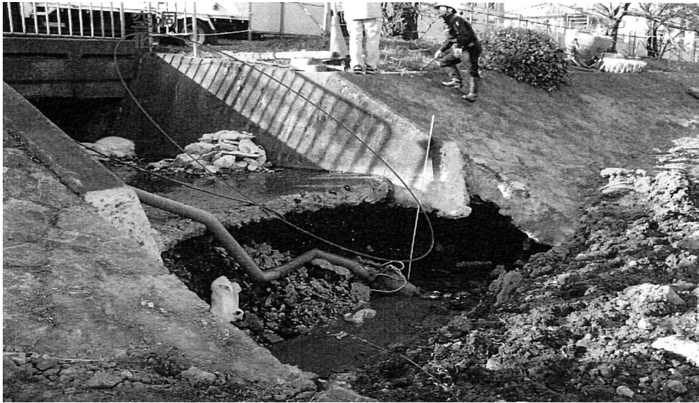
Figure 6.3 Erosion below the concrete face at the right side of the Seta River (January 2007)
