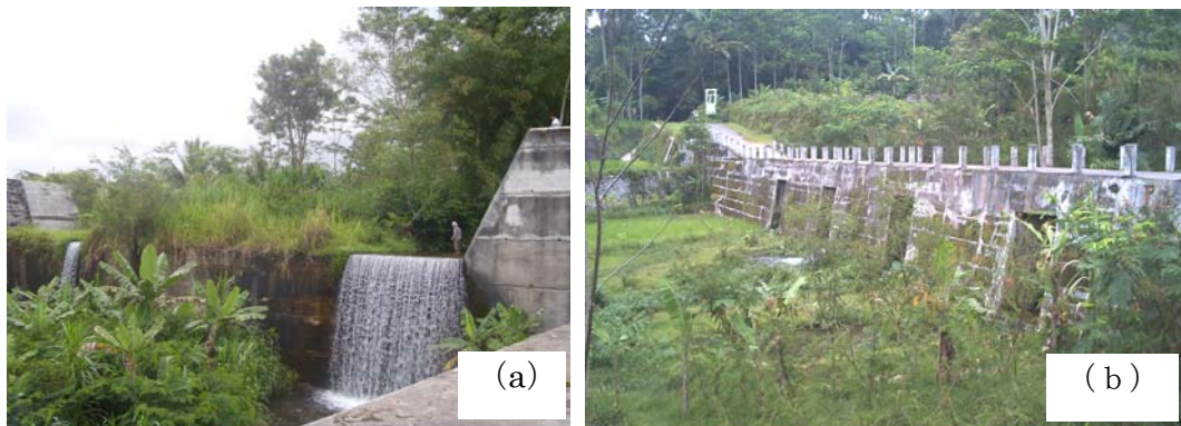
Photo 3.3 Existing of sabo works on slopes of Mount Merapi. (a) A Check dam functioned as an intake and a sand pocket on Blongkeng River (BLD1). (b) A Consolidation dam on Putih River functioned as a bridge (PU-C8A) (Photos were taken in December 2008)
