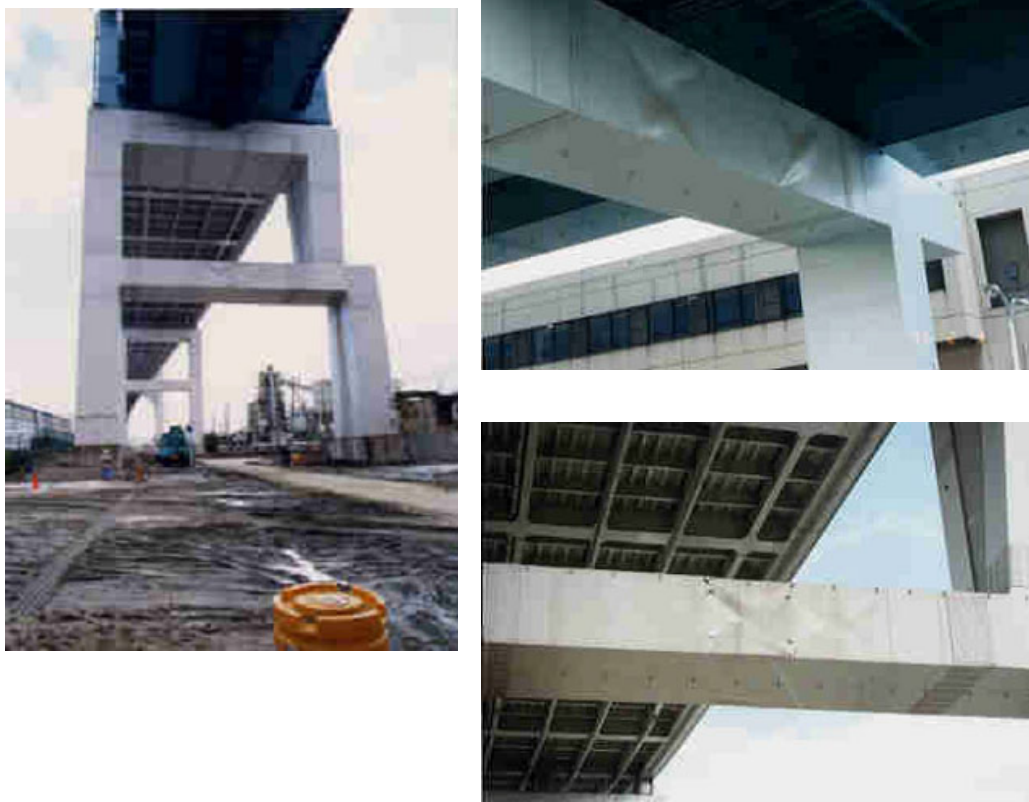
Fig.1 Shear buckling at box-beam in the Great Hanshin-Awaji earthquake
