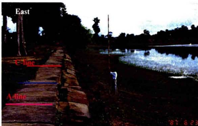
Photo 9-6 Leveling of steps of embankment at Srah Srang (see the location of Srah Srang in Fig.2-3)
