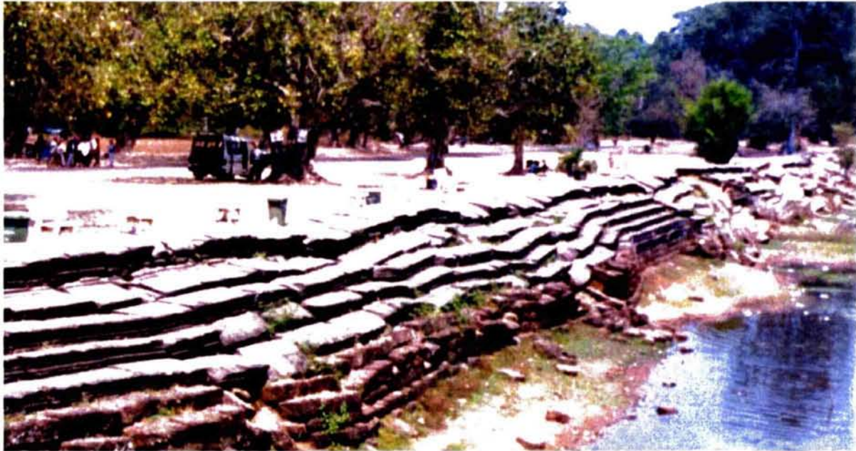
Photo 9-5 Inclination of embankment along moat of Angkor Wat
