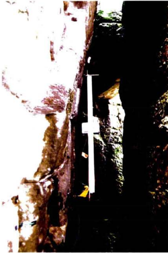
Photo 7-13 inclinometer installed on the Core Wall of Central Tower
