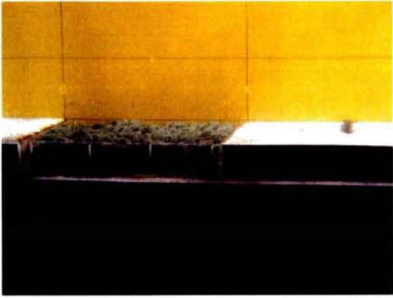
侵食状況 (C1-120)
