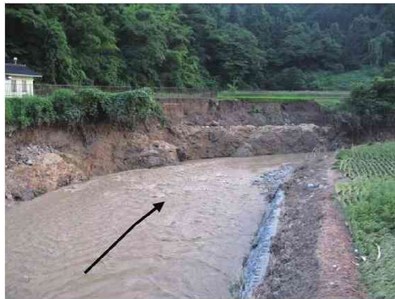
Fig.5 Erosion of outer river bank along meandering reach (taken on July 29)
