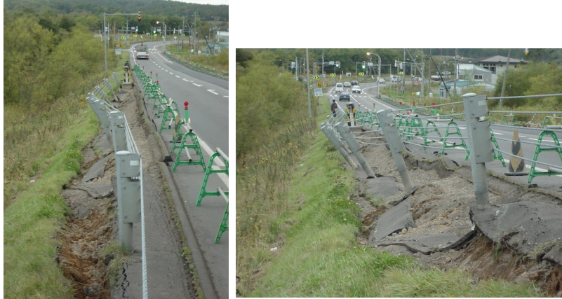
Figure 5.2 Shallow sliding failure in a road embankment in Chokubetsu, Onbetsu-cho during the 2003 Tokachi-oki Earthquake, Hokkaido, Japan (Yoshimine, 2003)
