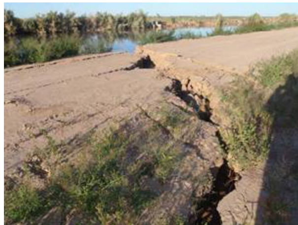
Figure 5.4 Transverse fracture offset the crest of the dike at the Westside Main Canal of the Alamo river during the 2010 Sierra El Mayor - Cucapah earthquake, Mexico (the GEER Association website)
