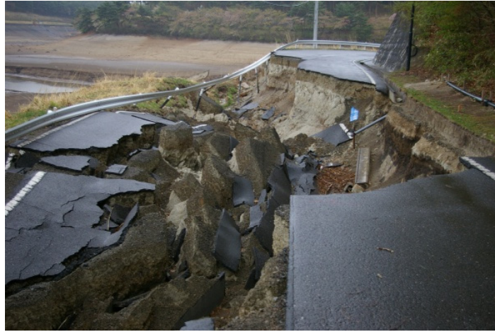
Figure 5.3 Deep sliding failure in a road embankment in Fukushima prefecture during the 2011 Tohoku Earthquake (Yoshimine, 2011)
