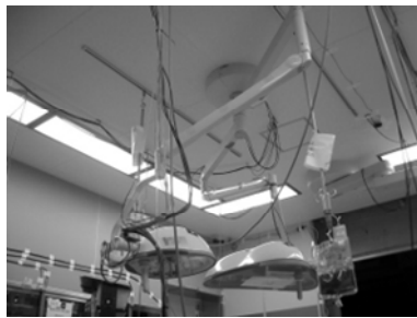
(a) Surgical light (Operating room)
