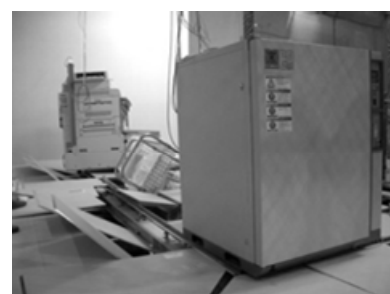
(c) raised floor panels
