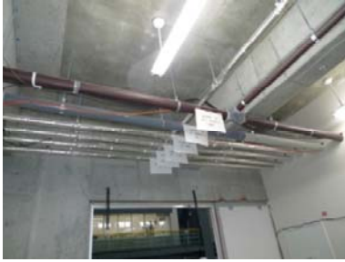
(a-2) Plumbing (Photo B)
