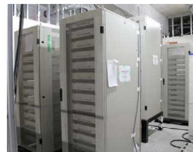
(b-3) Server room (Photo D)
