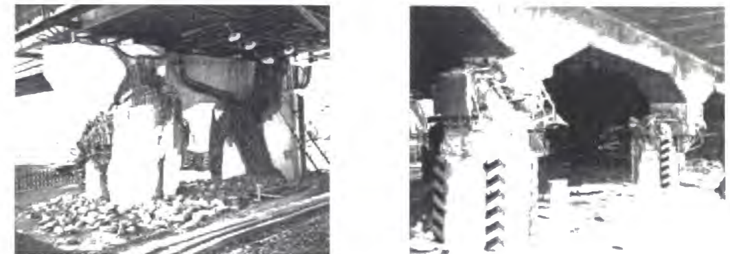
Figure 2.14 Damages to bridges in recent earthquakes
