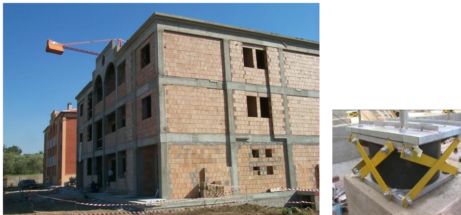
Figure 1.10 Three-story base isolated building with special mixed bearings (HDRB + Slider), Rapolla, Italy
