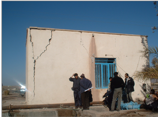
Fig 2.20 Damaged water deep well house
