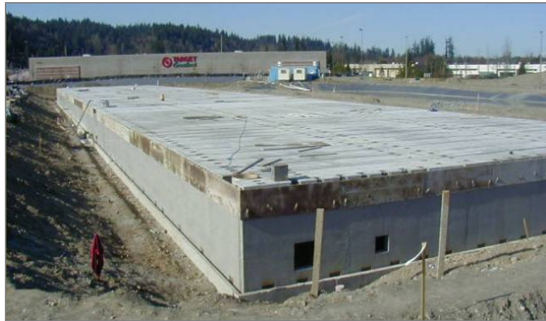
Fig 2.5 Reinforced water reservoir (elevated and at grade)
