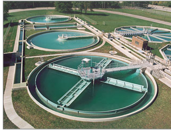
Fig 2.2 Water treatment plant (wetland)
