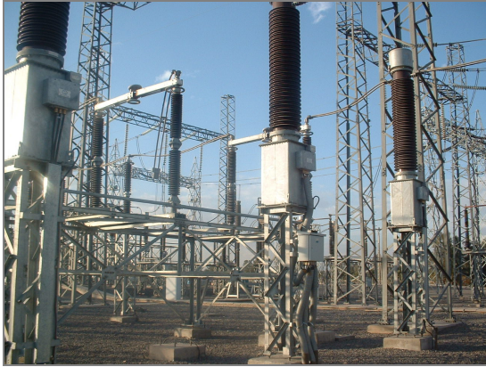
Fig 2.11 Power electric substation
