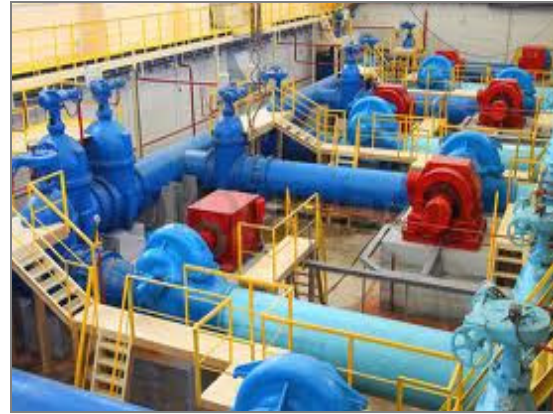
Fig 2.4 Pumps, piping and valves (colourbox)
