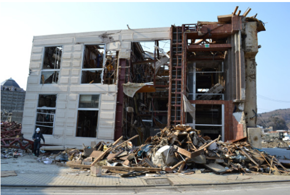
Photo 35 Toppled steel structure 4-story building F
