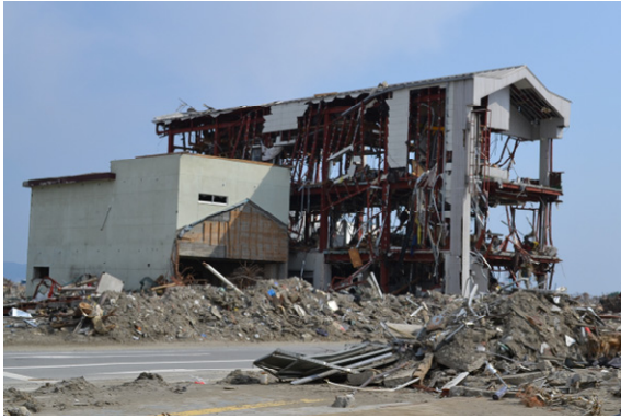
Photo 11 Damage to steel structure
