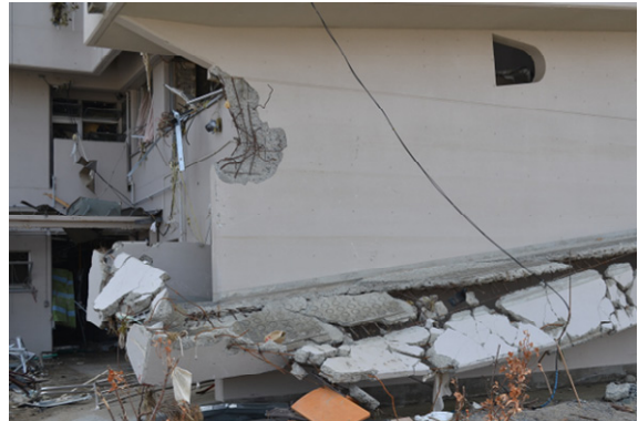
Photo 2 Damage to building A possible caused by floating wreckage
