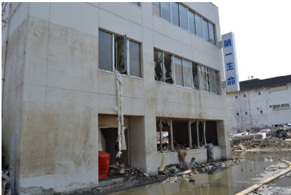
Photo 17 RC 3-story building, tsunami reached 2 nd floor
