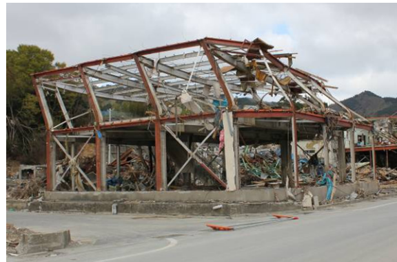
Photo 54 Damage to steel structure
