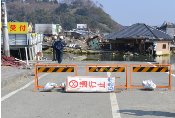
Photo 21 Road washed away by tsunami (Ishinomaki-city)
