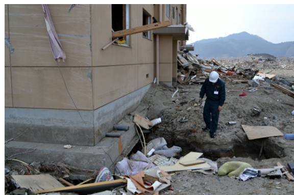
Photo 4 Scour around building B
