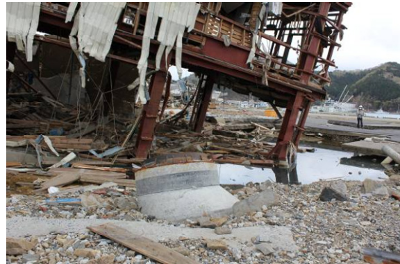
Photo 52 Extensive scour around building K
