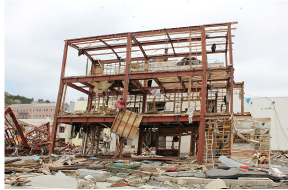
Photo 50 Damage to steel structure
