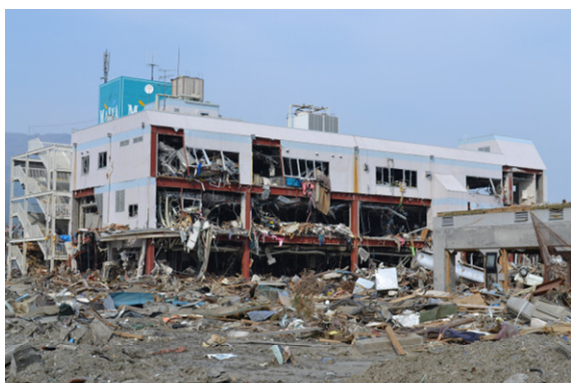
Photo 9 Damage of cladding of building D (Sea side)
