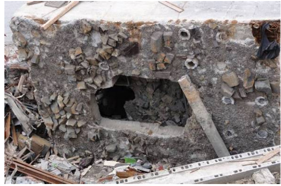
Photo 34 Pile of toppled building E
