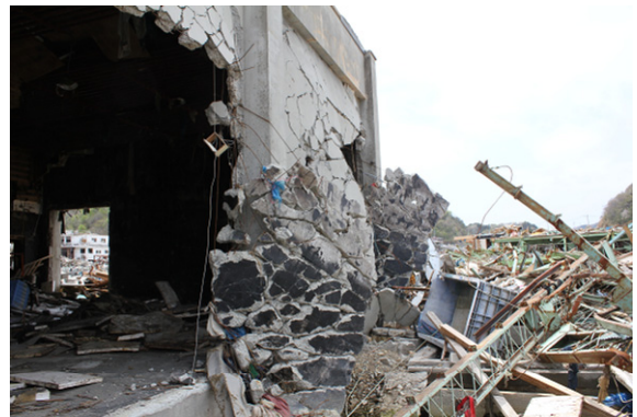
Photo 46 RC exterior walls out-of-plane failure
