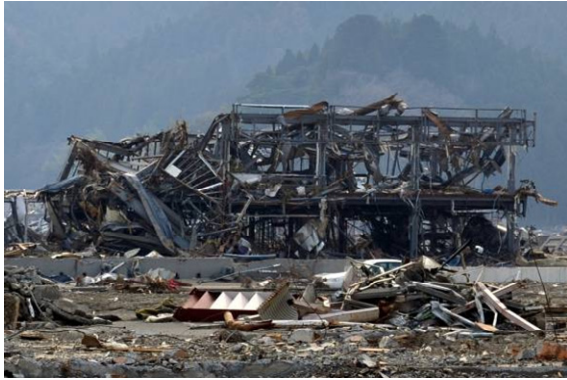
Photo 13 Damage to steel structure
