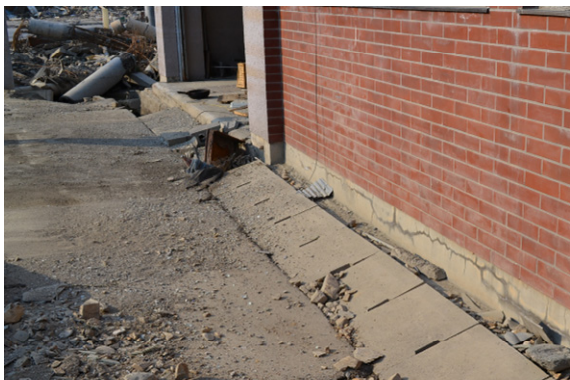
Photo 55 Ground settlement around building nearby building E
