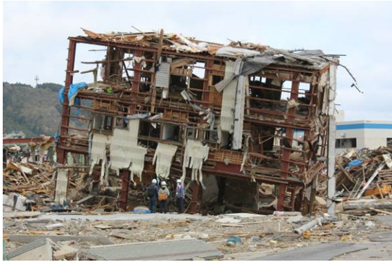
Photo 51 Tilted steel structure building K
