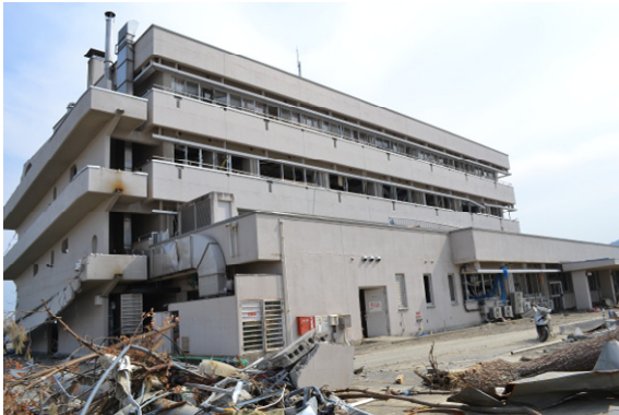
Photo 1 RC 4-story building A, tsunami reached 4th floor (Rikuzentakada-city)
