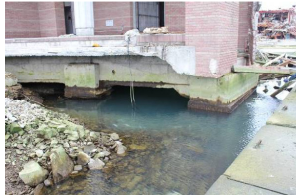
Photo 44 Extensive scour around building I
