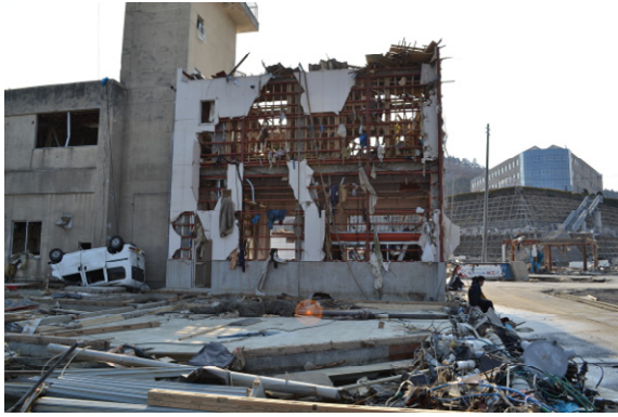
Photo 49 Damage to steel structure
