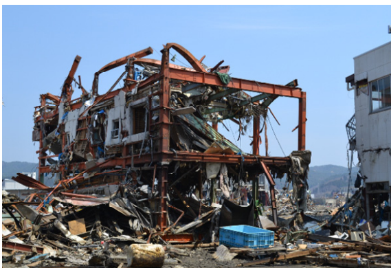
Photo 19 Damage to steel structure
