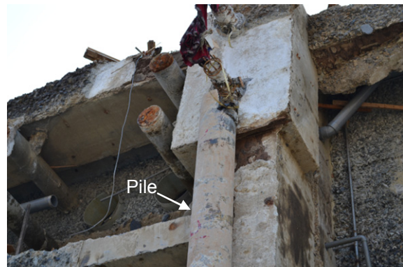
Photo 38 Pile of toppled building F
