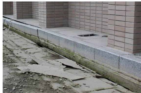
Photo 56 Ground settlement around building nearby building H
