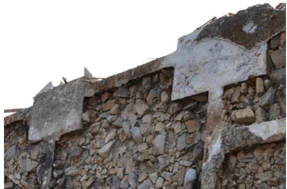
Photo 40 Pile cap of toppled building G
