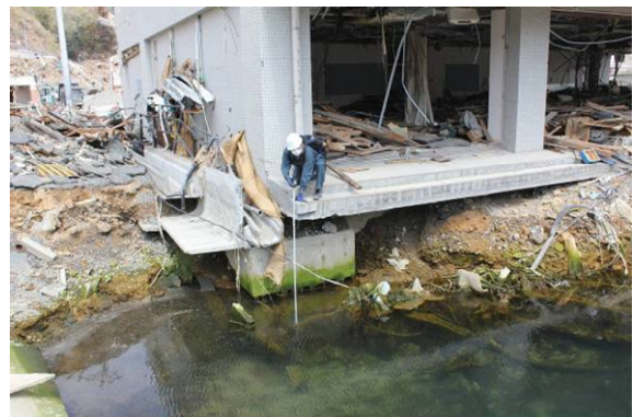
Photo 48 Extensive scour around building J
