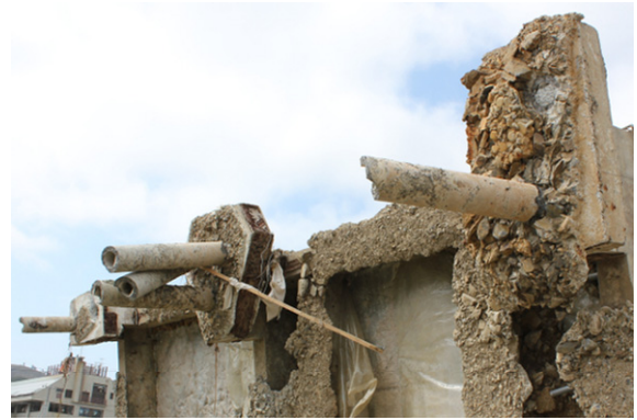
Photo 42 Piles of toppled building H
