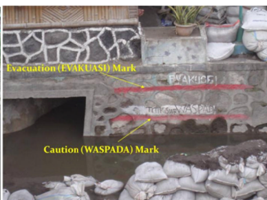
Photo 11 Community-based warning system in Code River
