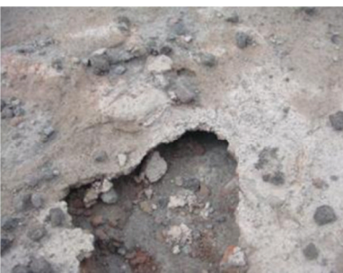
(b) Collapsed crust
