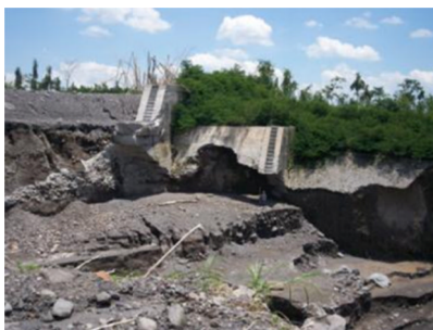
Photo 9(c) Collapse type 3
