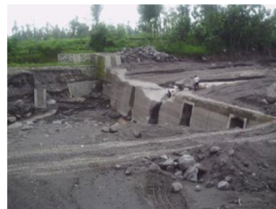
Photo 9(a) Collapse type 1
