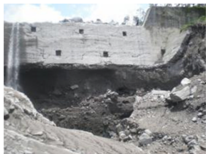
Photo 9(b) Collapse type 2
