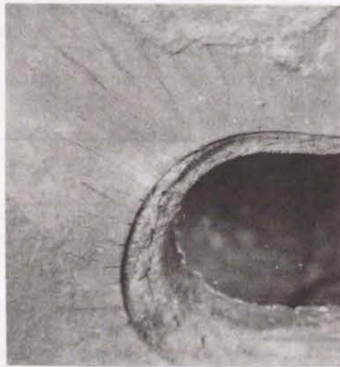
Fig. 9-35 An example of cracks found on the inner surface of the replaced steel shell
