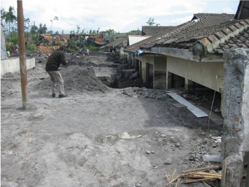
Fig. 3 Damage on houses near the volcanic river
