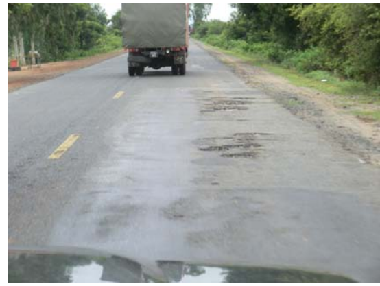
Fig. 1-2 Deterioration of DBST pavement
