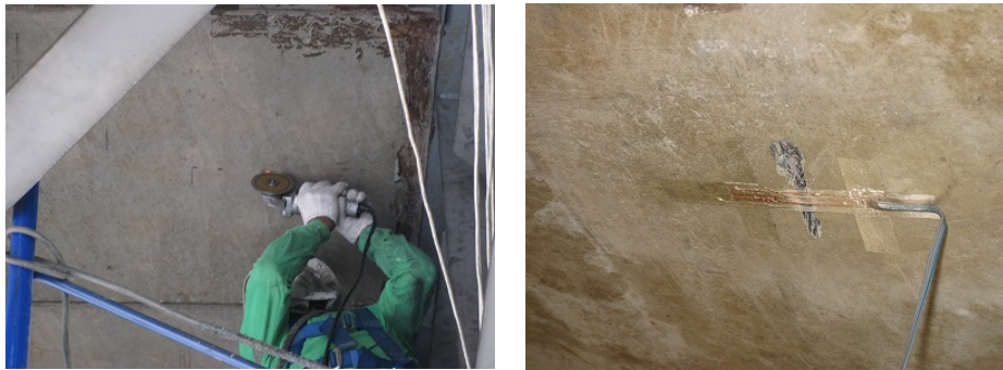
Fig. 5-6 Artificial crack by grinder on concrete slab
