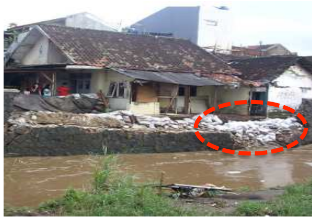
Figure 5.58: Man-made levee (from construction material) is destroyed due to riverine flood at Citepus River in Inhoftank area, Nyengseret Ward, Astanyar Sub-district, Bandung
