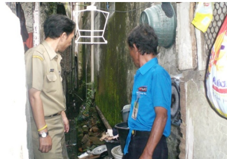
The leader of Community Information Group (KIM) Cibangkong Ward inspected the clogged gutter and drainage with a governmental officer
