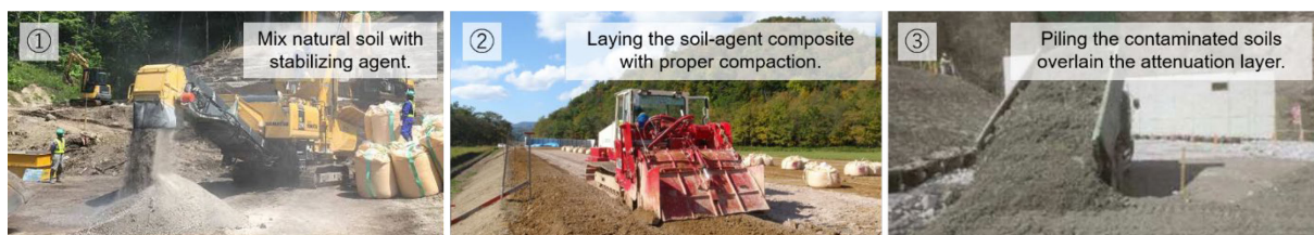
Figure 2.5: Representation of the construction process of the attenuation layer. Photo retrieved Feb 1, 2020, from https://cpds.kentsu.co.jp/technology/detail?id=40
