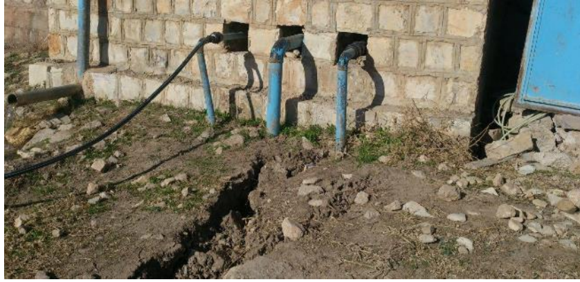
Fig. 1.7. Damage to the Gurchi-Bashi village vessel and Pipeline due to settlement and landslide in some parts.
