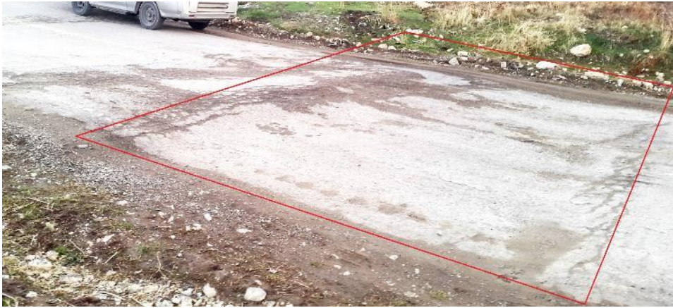
Fig. 1.4. Damage to village road nearby Sarpole-Zahab (the road has rehabilitated temporarily).
