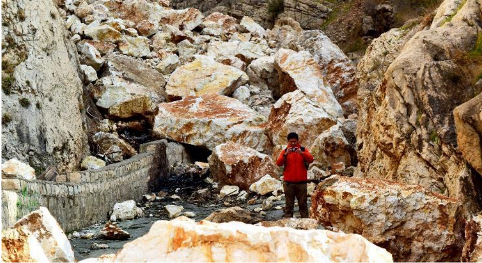
Fig. 1.3. Damage to Ban-Zardeg village road due to severe rock-fall.
