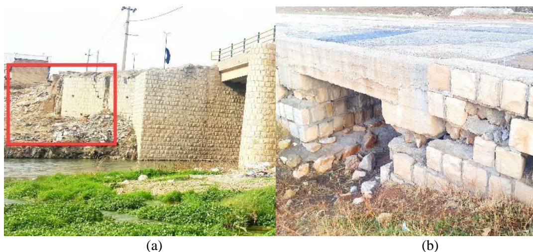
Fig. 1.2. (a) Damage to the retaining walls beside the bridge of Sarpole-Zahab City, (b) damage to little stone and concrete bridge at a Village road nearby Sarpole-Zahab [13].
