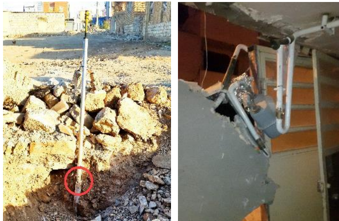
Fig. 1.8. Damage to joint of the gas pipeline at the entrance to the houses at Sarpole-Zahab city.
