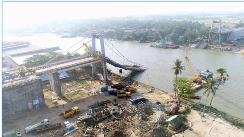
Figure 5.1 Myaungmya Bridge after collapse
