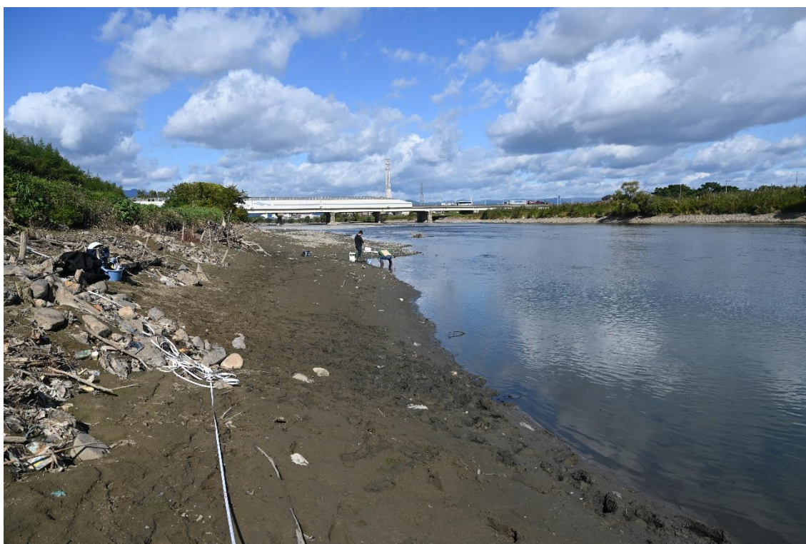
Fig. 5-8 Muddy layer along the right bank just upstream of No.1 weir.
