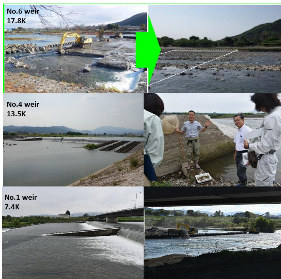
Fig. 4-3 Before and after (during) removal photos of No.6, No.4 and No.1 weir in Katsura River.
