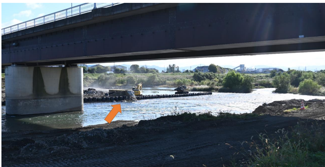
Fig. 5-2 During the removal of No.1 weir, the weir has been breached, and weir body was removing, the water level has been lowered and thus we can do field survey in the former impoundment area.
