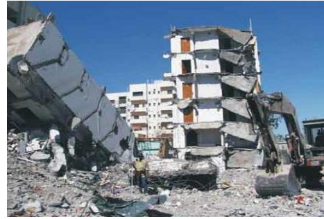
(b) Buildings damaged by 2001 Gujarat earthquake (Backhaus et al., 2010)
