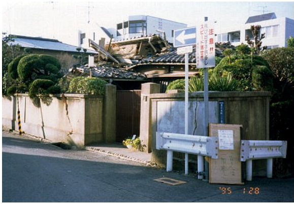
Photo 1 A collapsed wooden house (originally 2-storied) in Higashinada-Ward 11 days after the 1995 Hyogo-ken Nanbu (Kobe) earthquake (Photo by H. Kawase).
