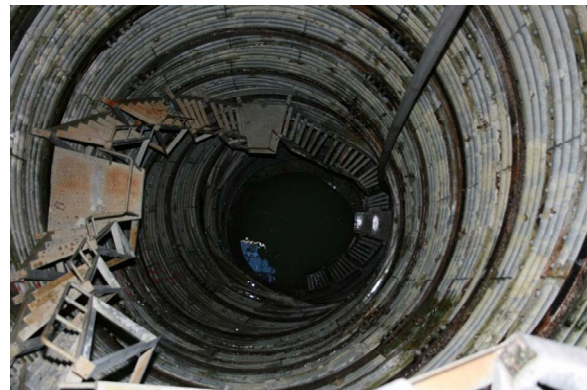
Fig. 15 Deformation and destruction of a drainage well in the accretionary prism landslides.
