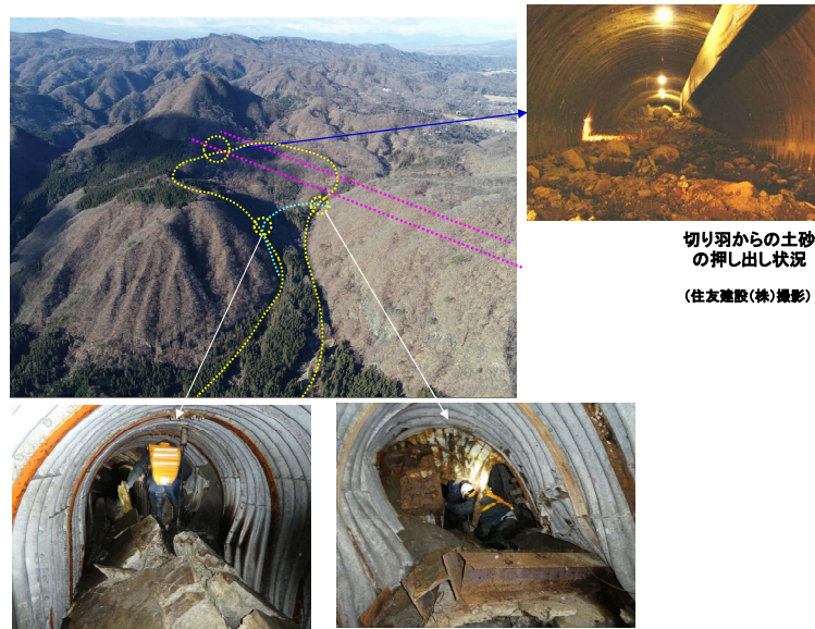
Fig. 14 Deformation and destruction of drainage tunnels due to landslide displacement.
