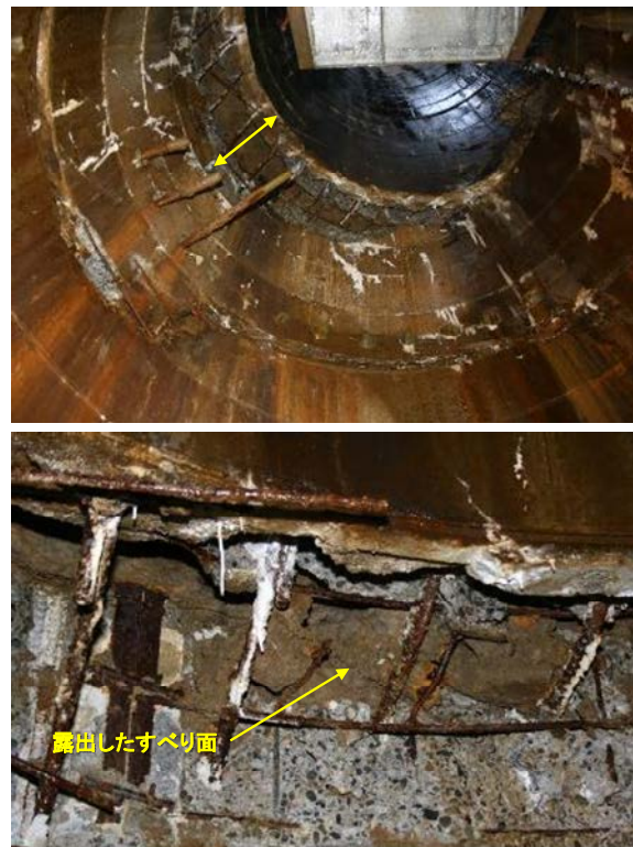
Fig. 13 Destruction of a concrete drainage well due to the displacement of reactivated landslide.
