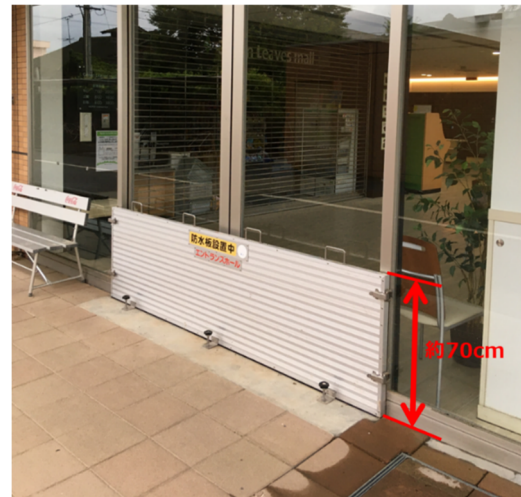
Photo 2 Installed water gate (July 23, 2020)
