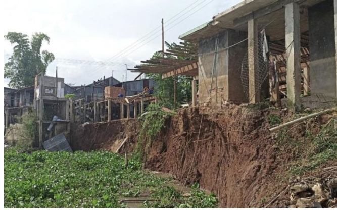
Figure 5.2 On June 5, 2021, at the bank erosion, is 90m long and 10-15m wide
