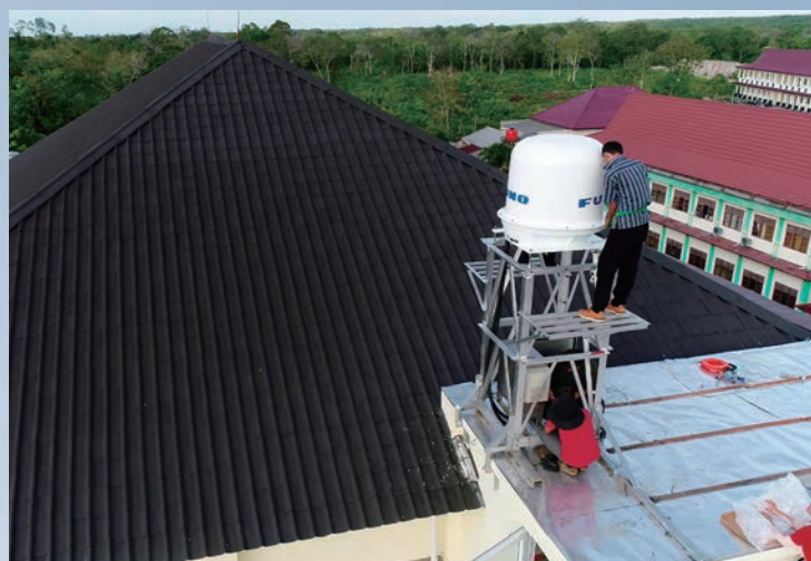
Photo 4 A weather radar device was installed in STAIN Bengkalis with the cooperation of both Furuno Electric engineers and the Agency for the Assessment and Application of Technology (BPPT). According to the facility staff, a forest fire occurred in the peatland behind the radar site in 2018. (Photo by Awaluddin, February 13, 2020)
