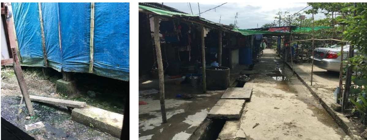
Figure 6.6 Water logging under the houses (Left) and drain in front of houses (Right)
