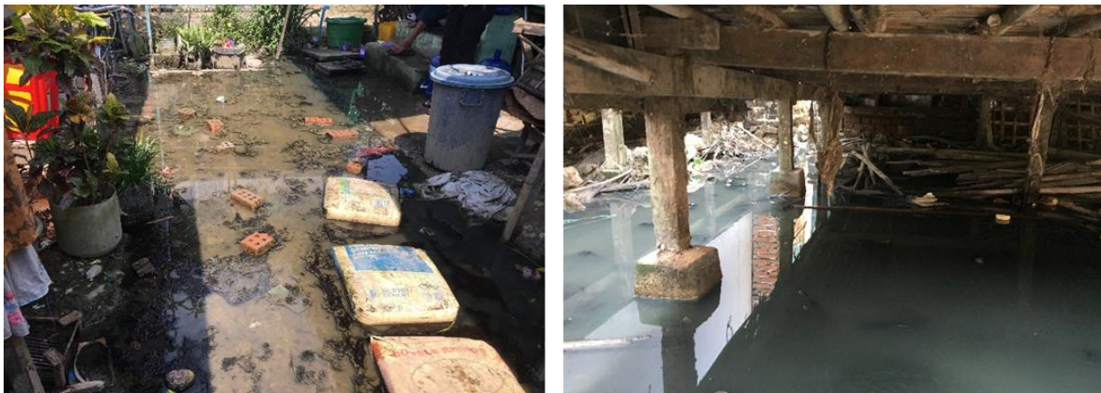
Figure 6.5 Water flooded on walking pathway (Left) and under the houses (Right)
