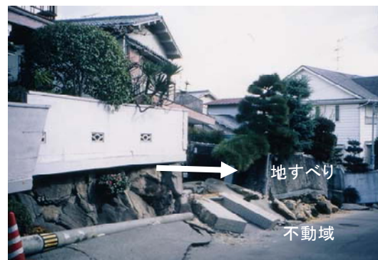
Photo 2 Landslide in residential valley fill in Nishinomiya City, caused by the 1995 earthquake
