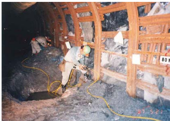
Photo 3 Installation of seismometers and cables near the fracture zone B in the survey tunnel excavated through the Mozumi-Sukenobe fault
