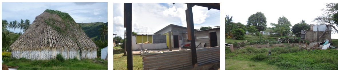
Figure 5. 14 (Left) Severely damaged and no longer liable in Site 2; (middle) severe but still liable house in Site 3 and (right) completely collapse house in Site 2 (Source: Mari Miyaji, Sainimere Veitata)
