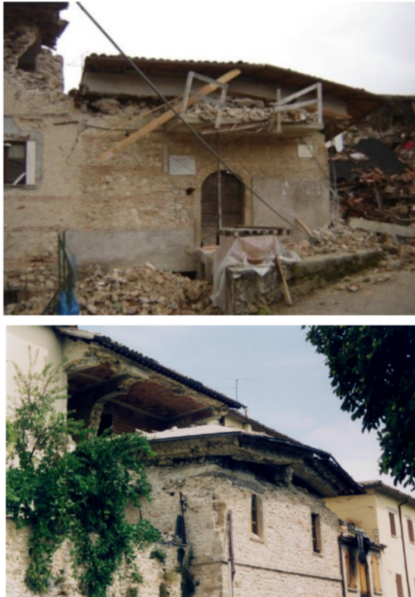
Figure 11: Damage due to roofing replacement [13].
