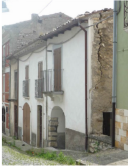
Figure 2: The mapping of the cracks that anticipates the vertical overturning of the wall [13].
