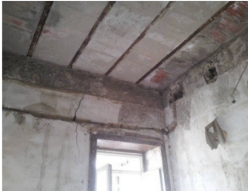
Figure 10: The crack in the masonry wall as a result of floor replacement with change of warping [13].
