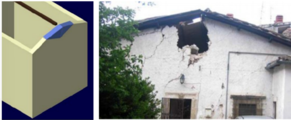
Figure 7: The gable collapse mechanism [13].
