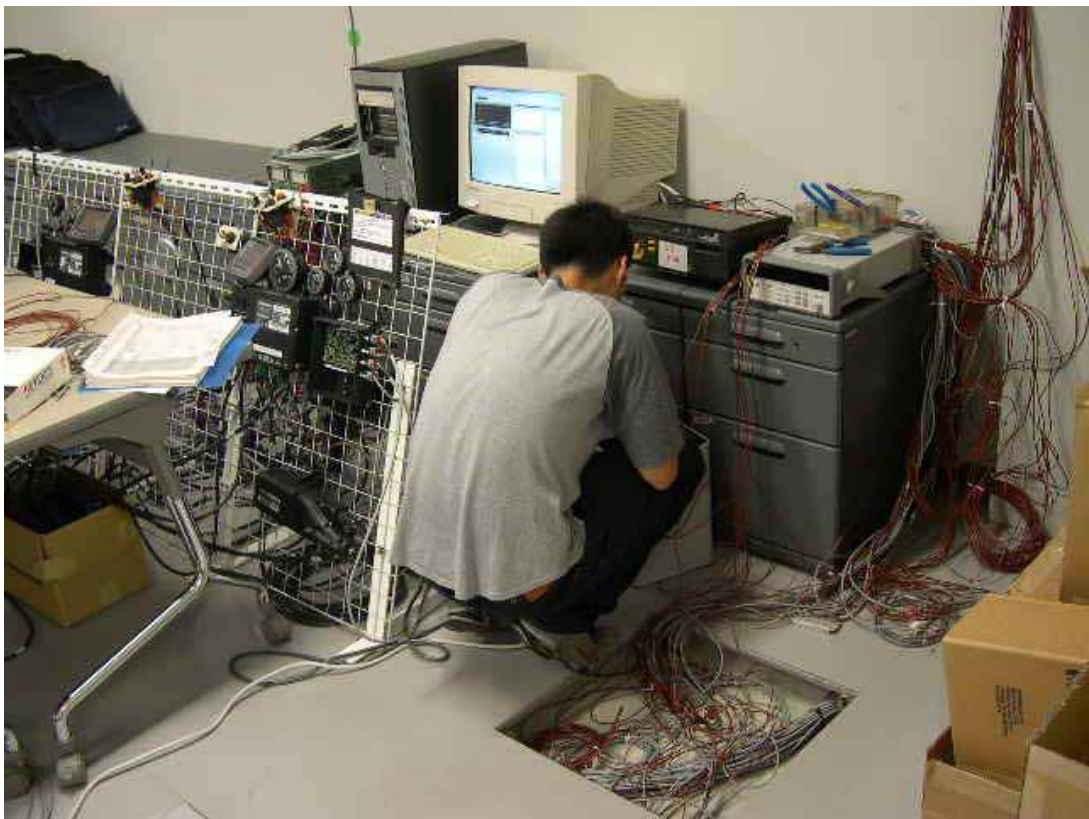
Figure A.16 Data loggers and wiring
