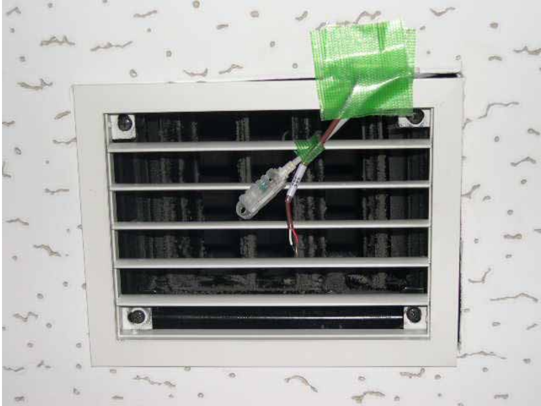
Figure A.15 Measurement of ventilation air temperature and humidity
