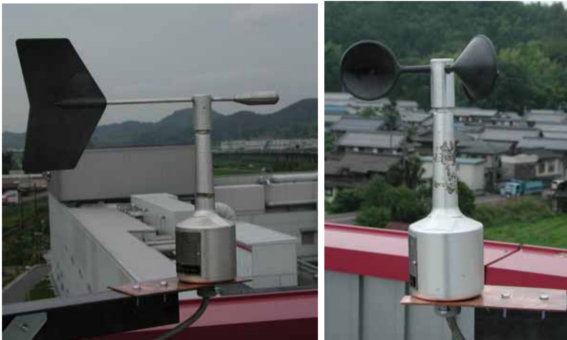
Figure A.4 Wind direction and speed measurement
