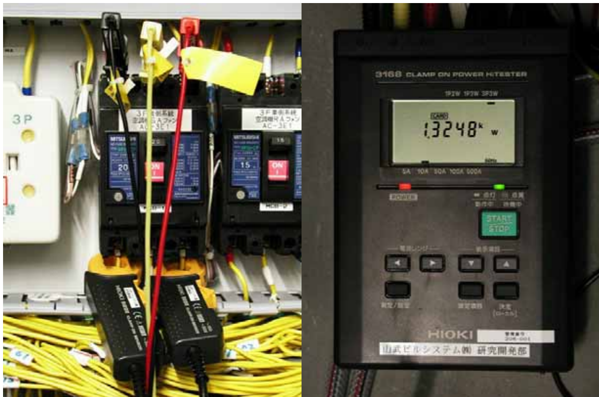
Figure 6.5 Power consumption measurement point and instrument
