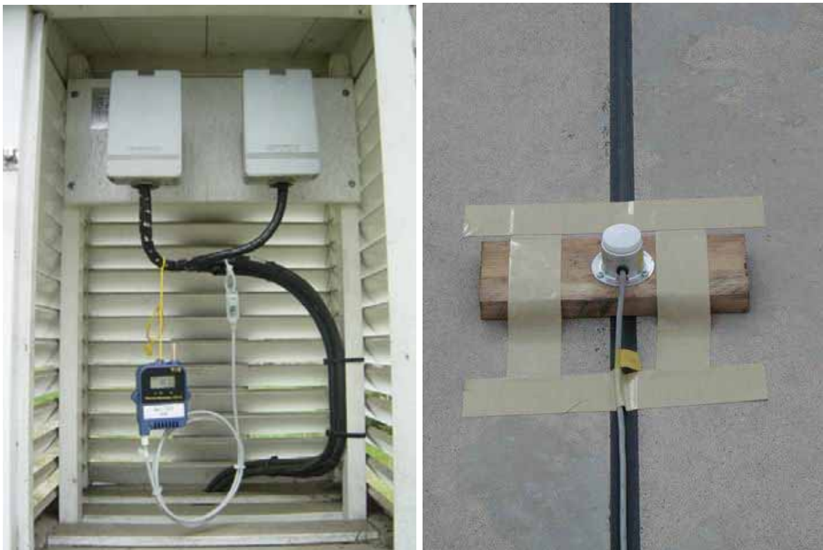
Figure A.3 Outdoor air temperature, humidity and solar radiation measurement
