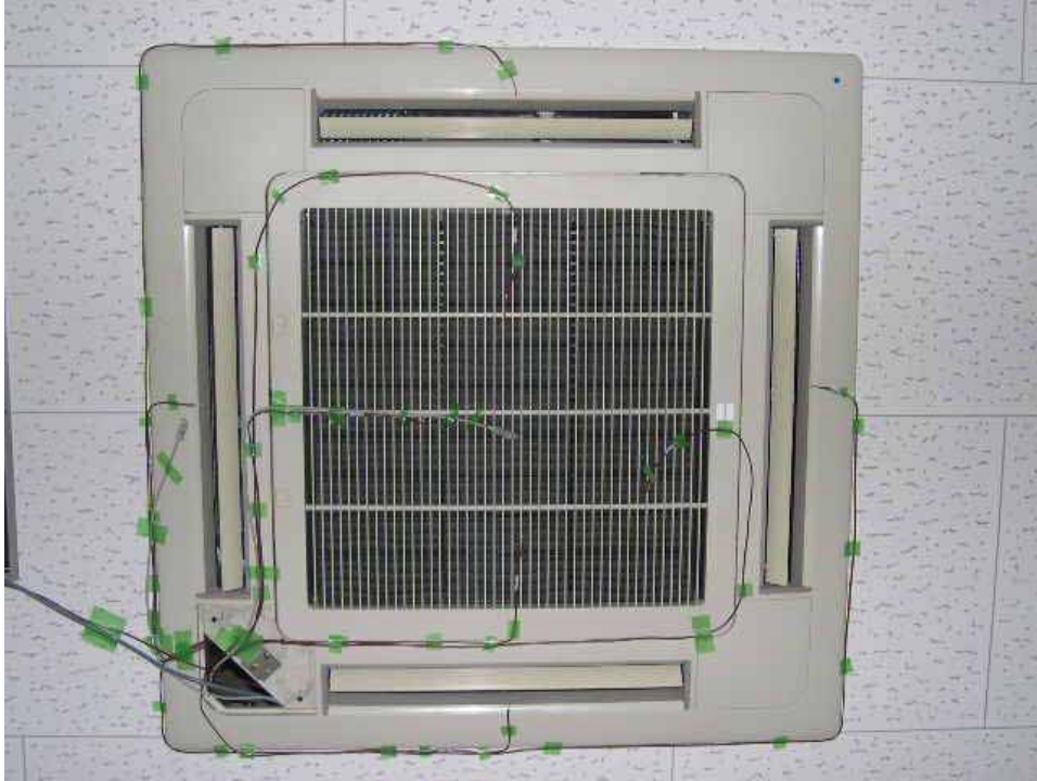
Figure A.8 Measurement of indoor unit inlet and outlet air temperature and humidity
