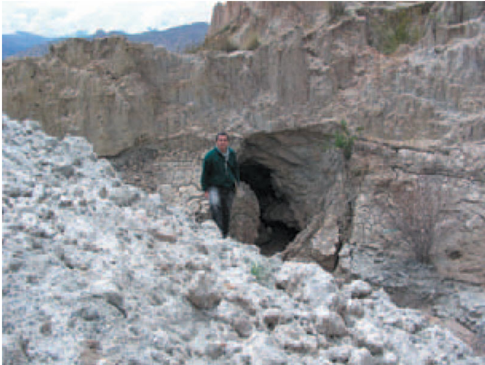
Figure 1.5 Natural water-escape tunnel through a landslide dam in Allpacoma valley, La Paz, Bolivia, formed due to piping failure.
