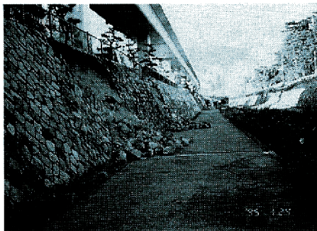
Photo 7 Collapse of stone revetment of Sumiyoshi River in Kobe
