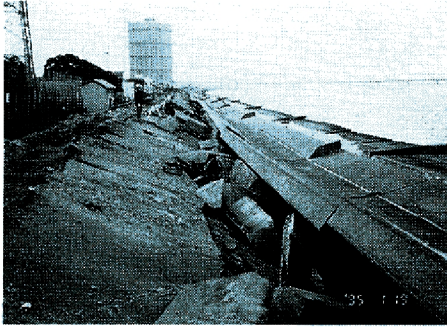
Photo 1 Perfectly collapsed embankment of Yodo River in Osaka
