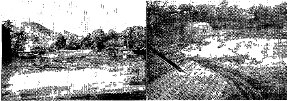
Photo 10 Collapse of the bank of Niteko reservoir
