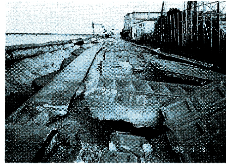
Photo 2 Perfectly collapsed embankment of Yodo River
