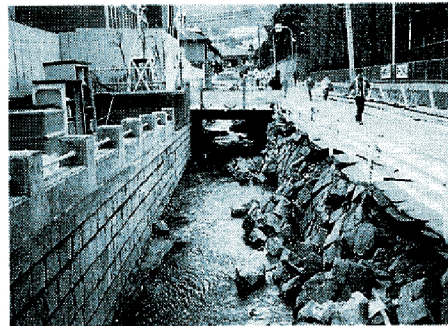
Photo 6 Collapse of stone revetment of Takaha River in Kobe
