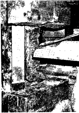
Photo 5 Repair detail observed at Warner Center Plaza #3
