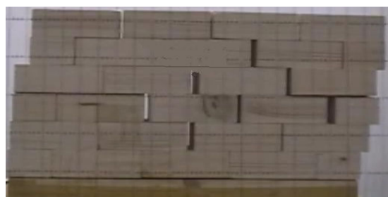
Fig. 5.6 deformed wood wall after experiment
