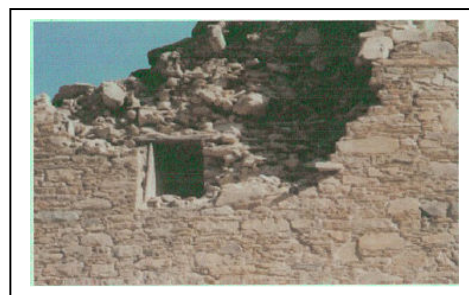
b. Delamination into layers
