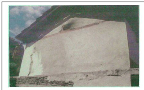
a. Corner cracking
