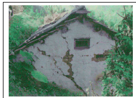
d. Racking shear failure
