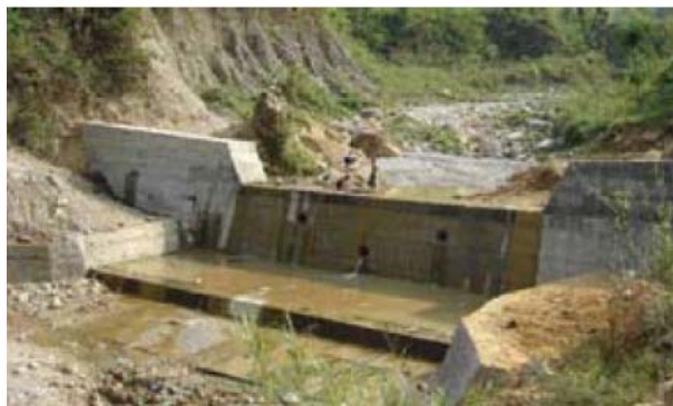
(c) Closed dam constructed at Khahare Khola stream in Muglin-Narayanghat Highway, Nepal (Source: Department of Water-Induced Disaster Prevention, Nepal)
