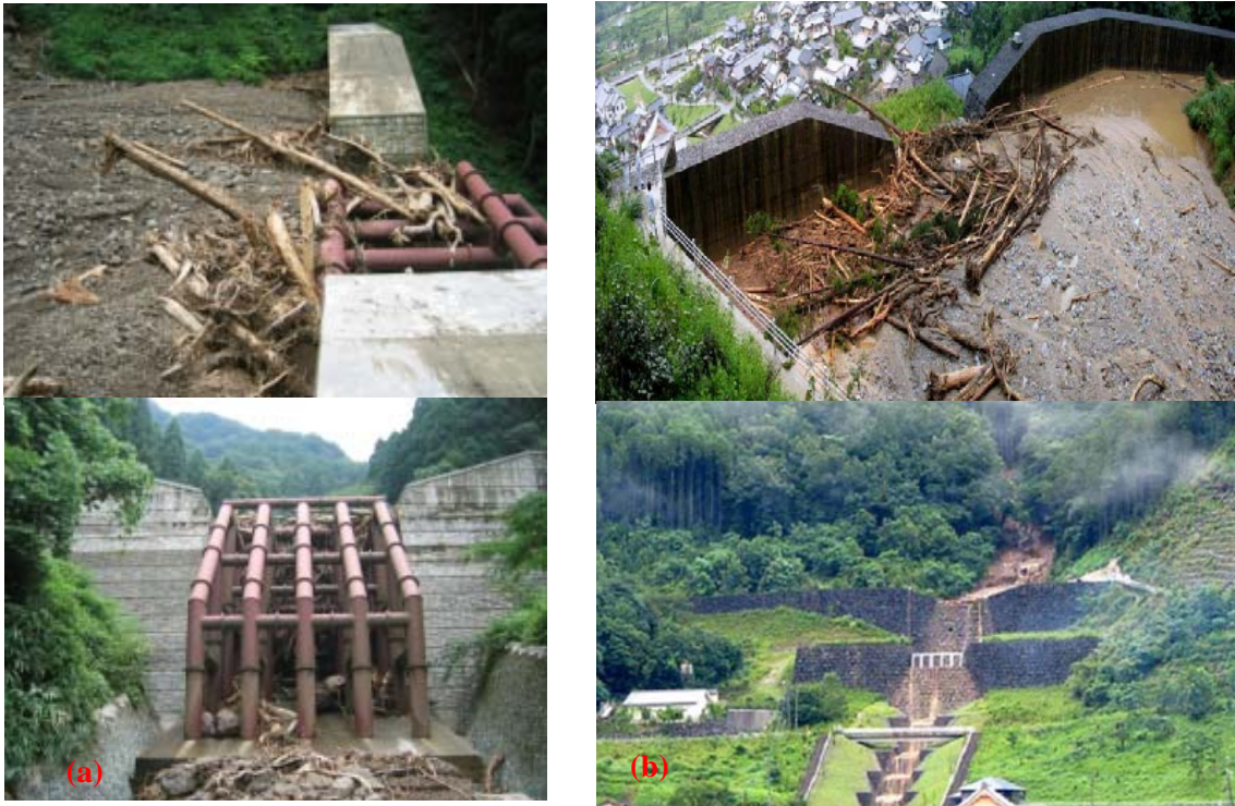
Figure 1.15 (a) Debris flow and driftwood captured by grid dam at the Mae Tanikawa River, Fukui Prefecture, Japan, 18 July, 2004, (b) Sabo dam trapped about 6000m 3 debris flow and driftwood at the Kawabegawa River, Kumamoto Prefecture, Japan, 24 July, 2006 (Photo Courtesy: Sabo Department, MLIT, Japan)
