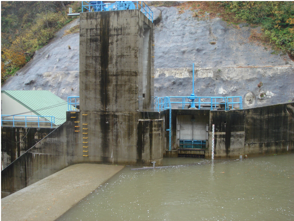
Figure 6.8: Intake at the Okumotani power station
