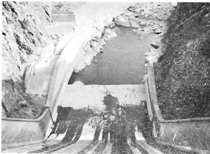
Fig. 15. Erosion at Nagayasuguchi Dam.
