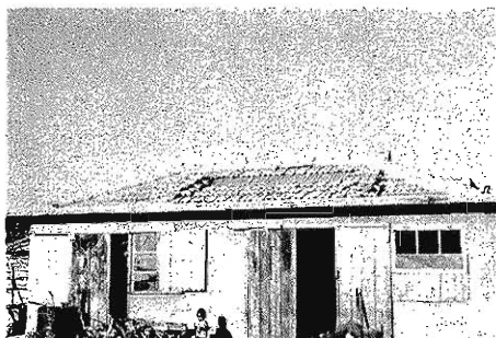
Photo. 8 Damage to a cement-tile roofing : tiles were removed extensively from the roof (damaged part are repaired by sheet-zincs).
