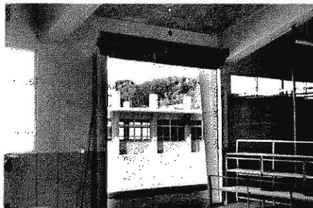
Photo. 6 Damage to light-gauge steel shutter : complete removal of shutter from the opening.
