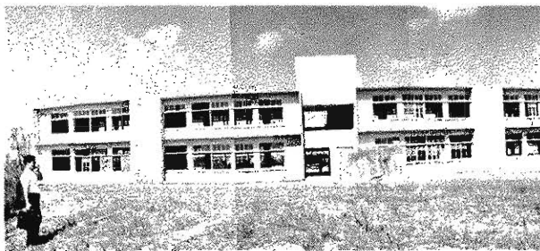
Photo. 4 Damage to a wooden school building : removal of wooden sashes from windows.
