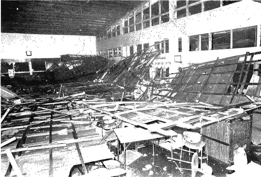
Photo. 4. Damage to a steel structure. Complete removal of the roof and collapse of the ceiling. (by courtesy of the Chunichi Newspapers)
