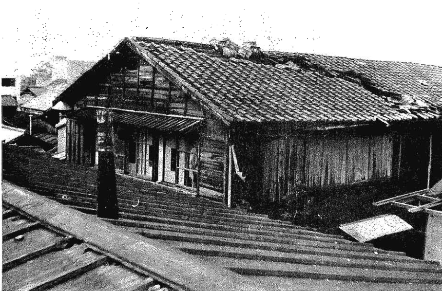
Photo. 5. Local damage to a tiled roof caused by heavy debris. (by courtesy of Mr. K. Chikada)
