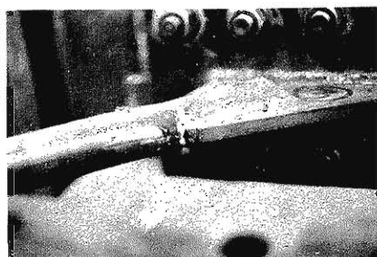
Photo. 8. Crack Initiation at the Edge of Gusset Plate.
