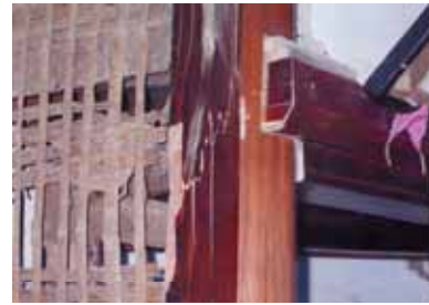
Fig.16 Break of column (NMH)
