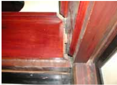
Fig.14 Separation of lintel-column joint (YIY)
