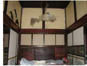
Fig.13 Cracks in hanging wall (YIY)
