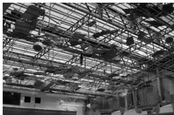
Photo 6. Blow off of a gymnasium roof.
