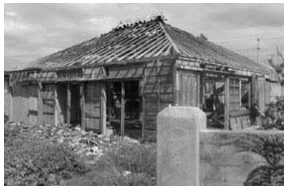
Photo 5. Completely destroyed wooden house.
