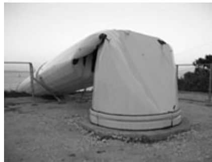
fallen tower of wind turbine
