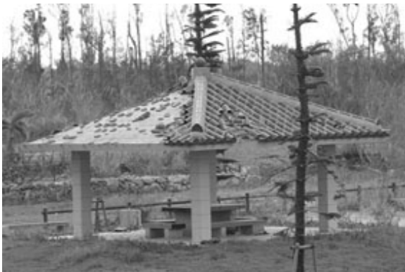
Photo 8. Blown off damage to the roof tiles of summerhouse
