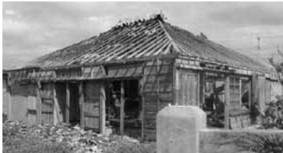
Photo 1 Completely destroyed wooden house
