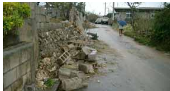
Photo 12 Fall down of concrete block wall (courtesy Miyakojima local weather station)
