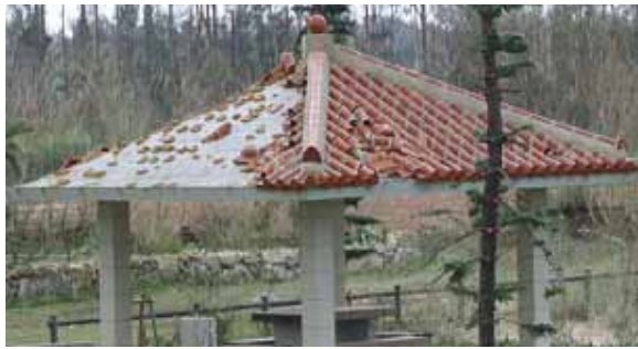
Photo 7 Roof tile damage of summer house
