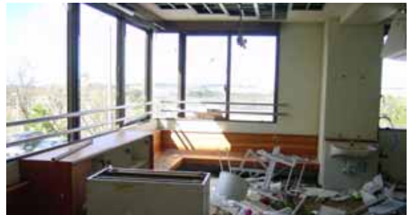
Photo 4 Interior damage with window breaks ( courtesy Okinawa Prefecture branch office )
