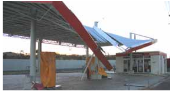
Photo 8 Roof damage of gas station (courtesy Kajimakensetu)
