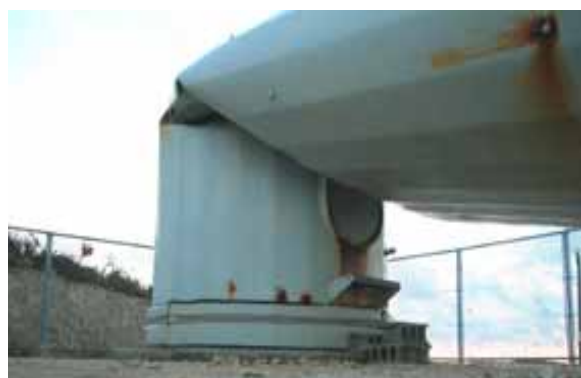
Photo 23 Tower was bended down at maintenance hatch (courtesy Kajimakensetu)
