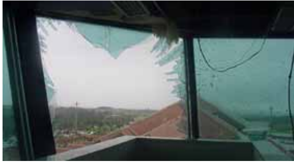
Photo 29 Window breaks at control tower of Miyakojima airport ( courtesy Okinawa Prefecture )
