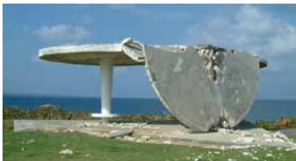
Photo 13 Damage of observation deck (courtesy Hirara city)
