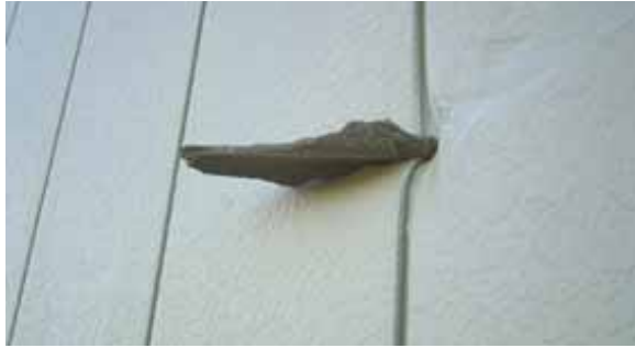
Photo 28 A piece of slate stuck into wall ( courtesy Building Research Institute )
