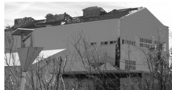
Photo 6 Damage of a sugar factory ( Okuda et. al., 2003 )
