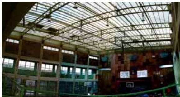
Photo 5 Damage of gymnasium ( courtesy Okinawa Prefecture branch office )
