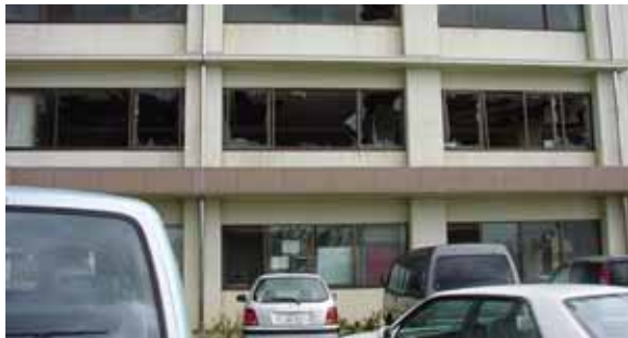
Photo 3 Damage of openings ( courtesy Okinawa Prefecture )
