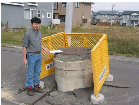
Fig. 1 Observed uplifted manhole after 2003 Tokachi-oki, Japan, earthquake.
